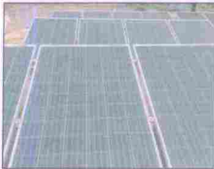
Photograph of Roof Top Solar PV Plant:
