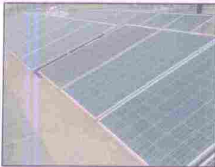
Photograph of Roof Top Solar PV Plant:
