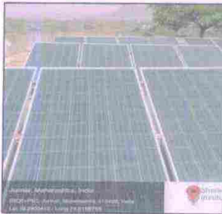
Photograph of Roof Top Solar PV Plant:
