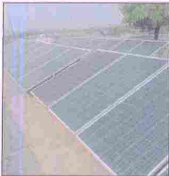
Photograph of Roof Top Solar PV Plant:
