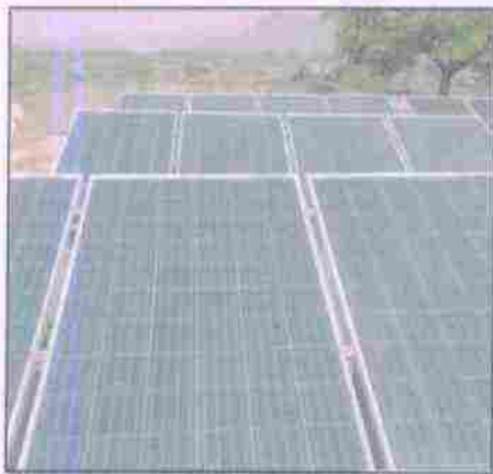
Photograph of Roof Top Solar PV Plant:
