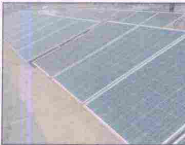
Photograph of Roof Top Solar PV Plant:
